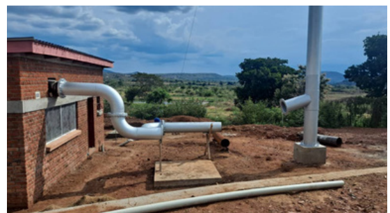
Mutambara Mission Hospital Incinerator
