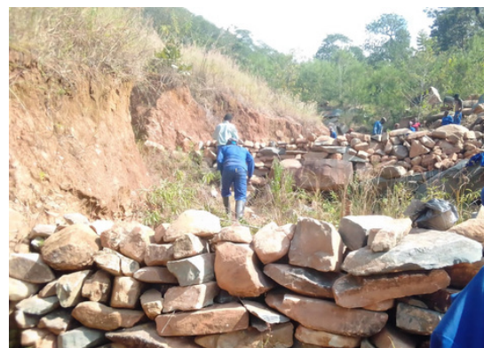
Top right: Farmers laying pipes from wells to water points at Musasa Microwatershed Bottom: Farmers constructing leaky weirs
